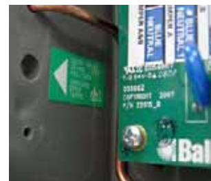
Ground in System Enclosure
