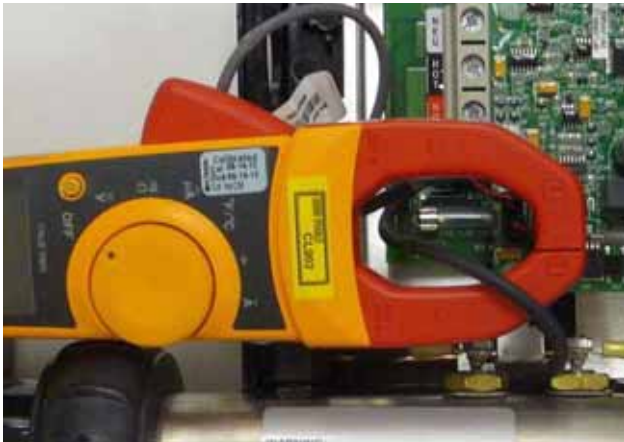
AMPERAGE HEATER TEST BP600
